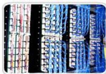
UTP patch panels in a rack
